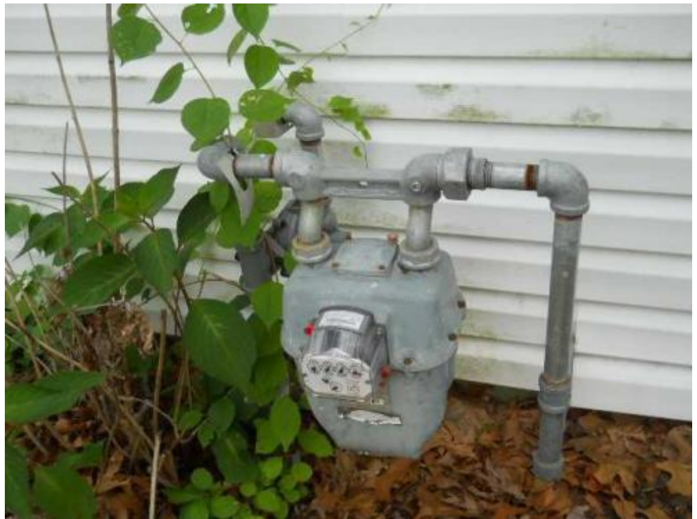
12 gas meter Date Taken: 7/21/2014 Taken By: Brook Benvenuti
