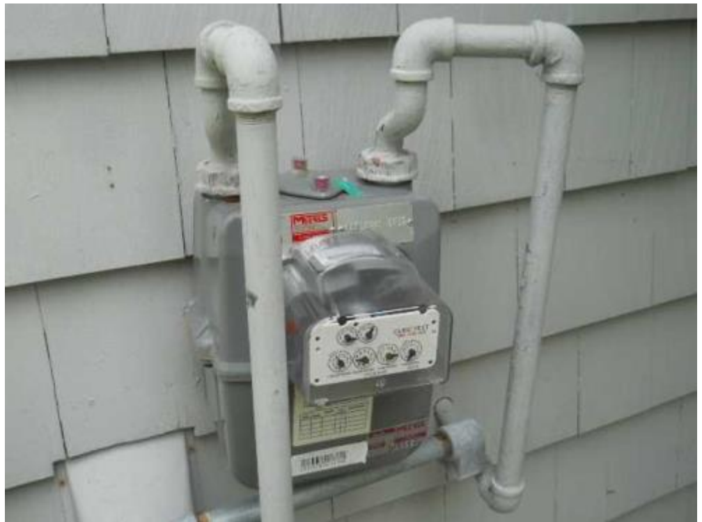
18 gas meter Date Taken: 7/21/2014 Taken By: Brook Benvenuti
