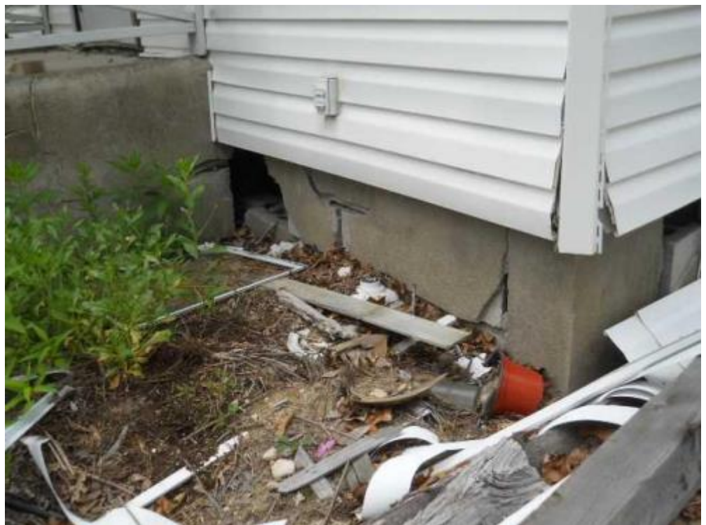
22 foundation damage Date Taken: 7/21/2014 Taken By: Brook Benvenuti
