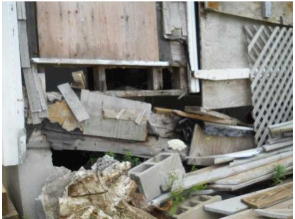
18 rear damage Date Taken: 7/21/2014 Taken By: Brook Benvenuti
