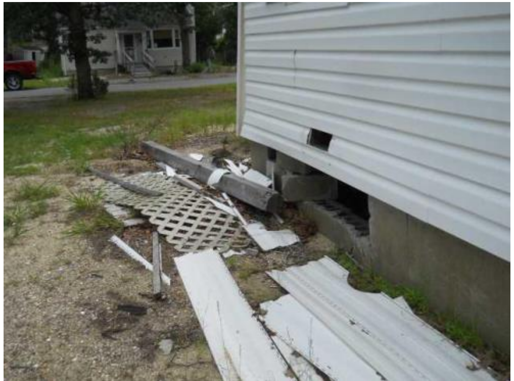
21 right debris Date Taken: 7/21/2014 Taken By: Brook Benvenuti
