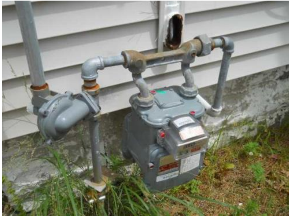
17 gas meter Date Taken: 7/21/2014 Taken By: Brook Benvenuti
