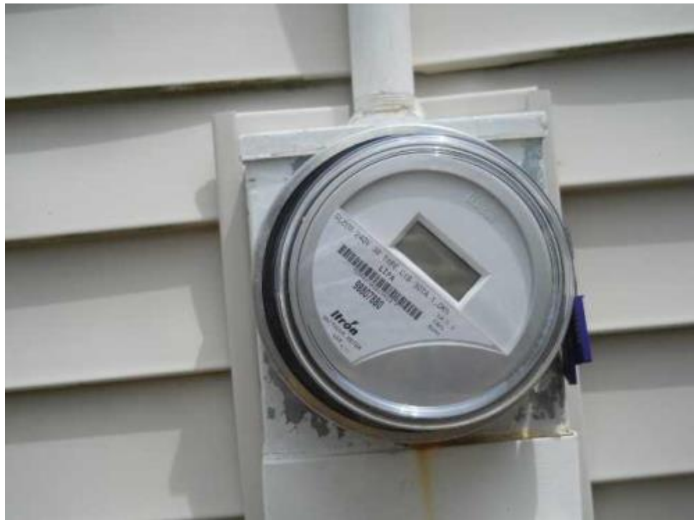
18 electric meter Date Taken: 7/21/2014 Taken By: Brook Benvenuti
