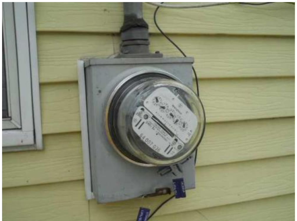
16 power meter Date Taken: 7/21/2014 Taken By: Brook Benvenuti
