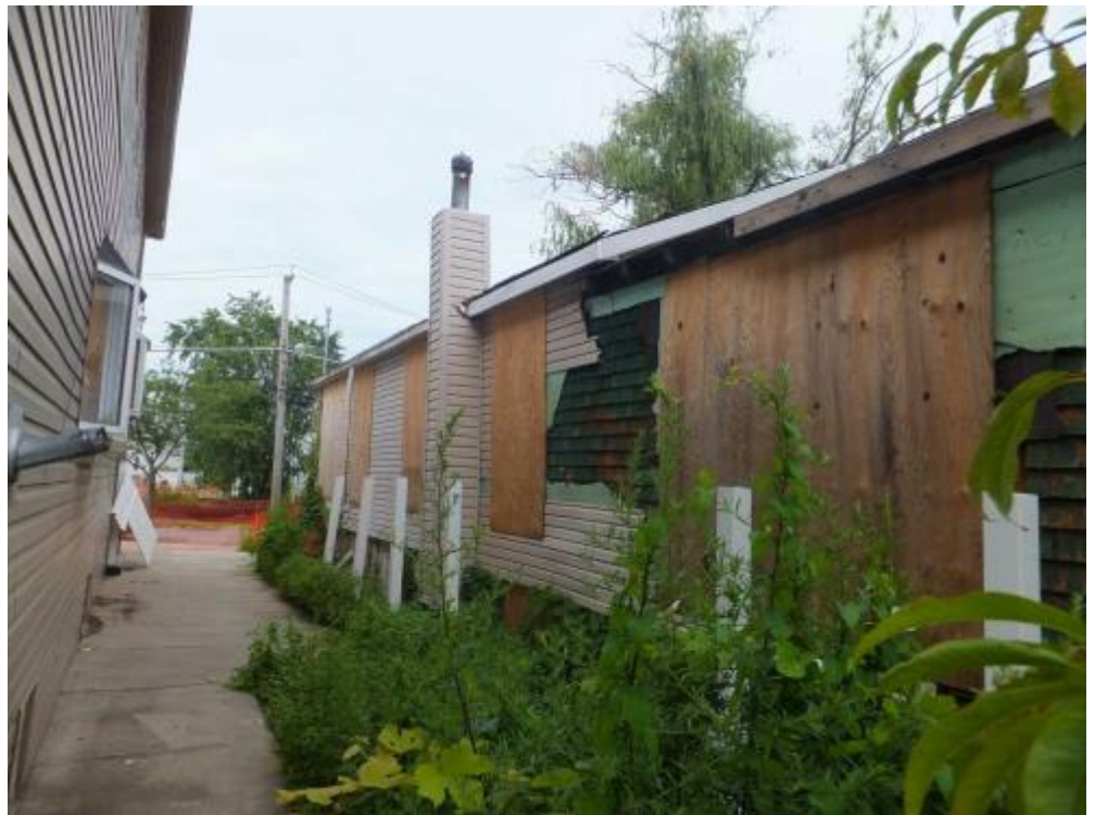
16 Right-Elevation Date Taken: 7/19/2014 Taken By: MGREEN Back to front view of the right side of the of the elevation. Shows damaged siding and overgrown vegetation.
