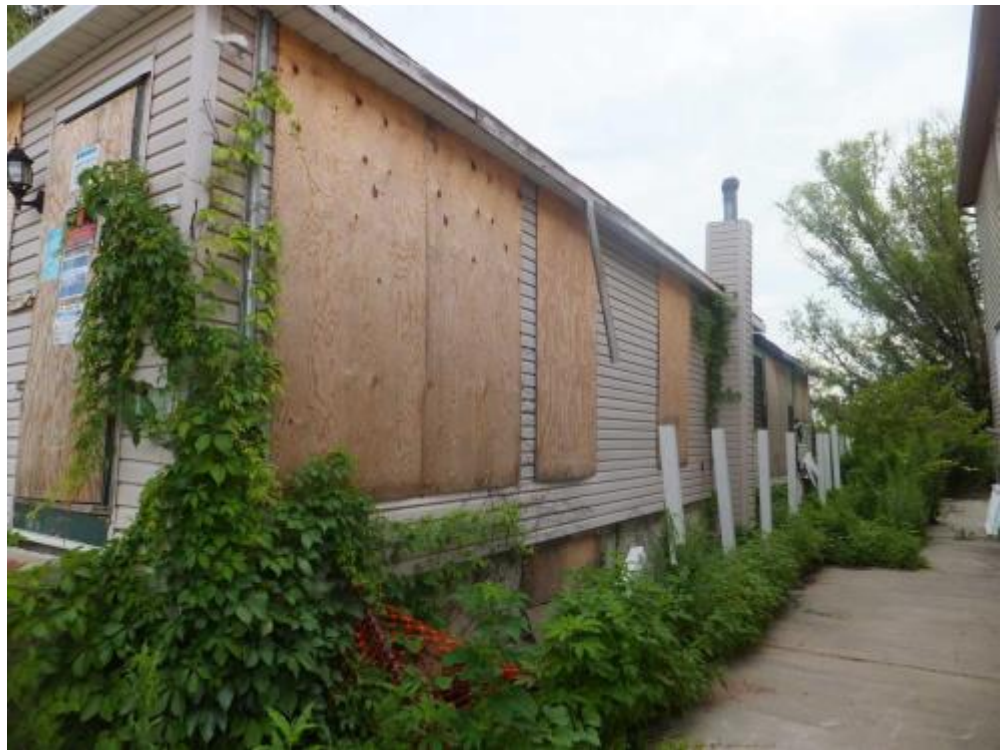
12 Right-Elevation Date Taken: 7/19/2014 Taken By: MGREEN Overall view of right elevation. Shows overgrown vegetation and boarded up windows.
