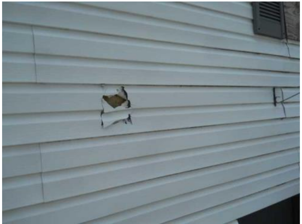
14 rear damage Date Taken: 7/16/2014 Taken By: Brook Benvenuti
