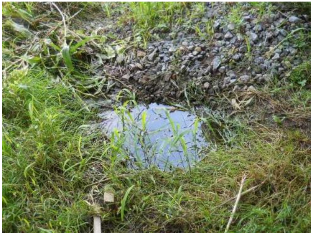
20 standing water Date Taken: 7/19/2014 Taken By: Brook Benvenuti
