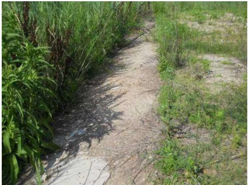
10 concrete slab Date Taken: 7/19/2014 Taken By: Brook Benvenuti
