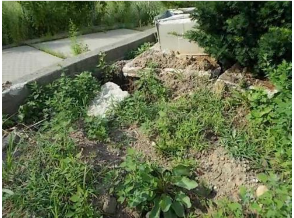
15 Back yard Date Taken: 7/18/2014 Taken By: Cham Benvenutti Uneven ground, holes and debris
